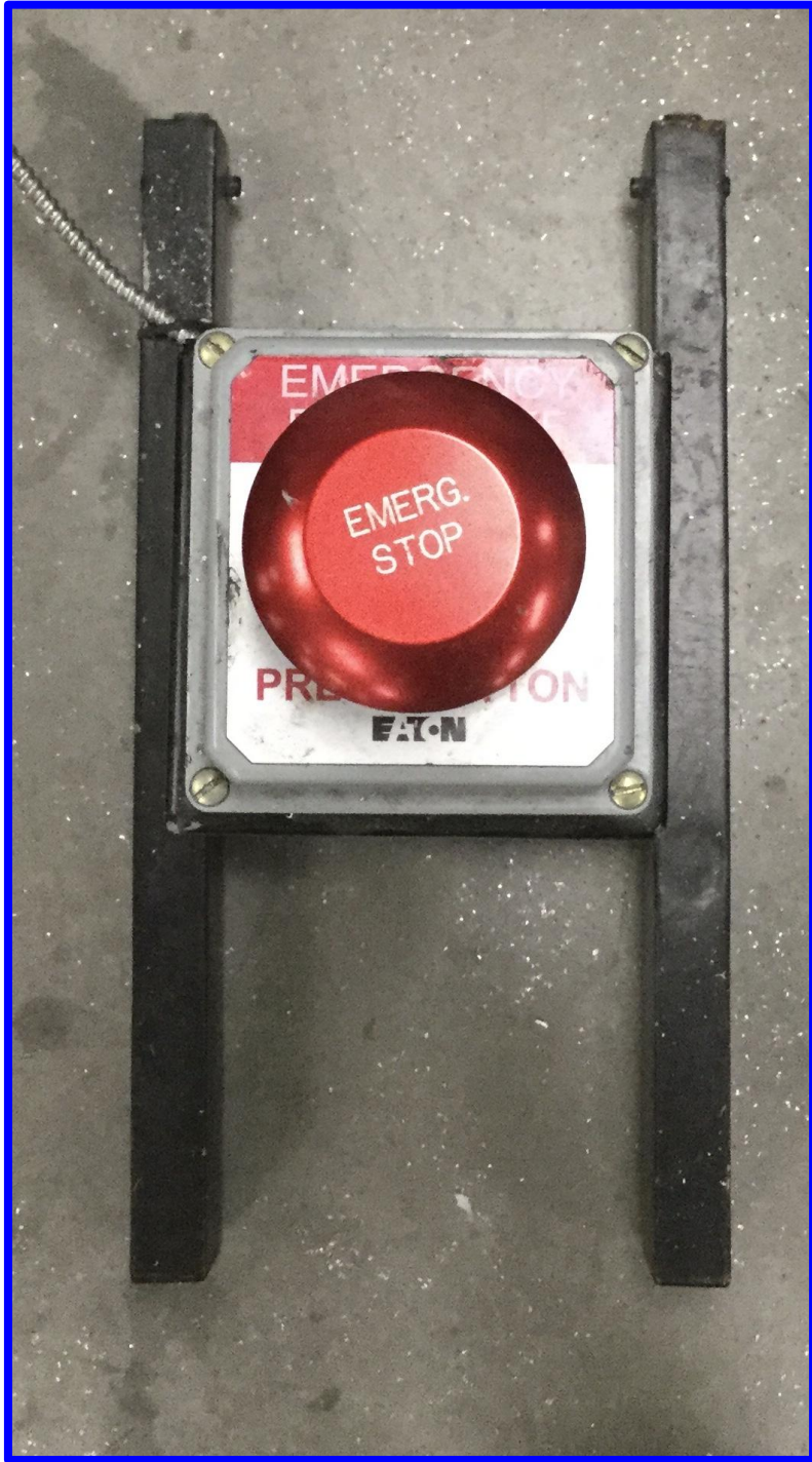
Emergency stop button for the mill
